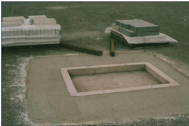
A precast slab with four-5" thick containment walls was placed in the asphalt parking lot. The paving area was 36½" x 54". The slab below the pavers was four inches thick.
