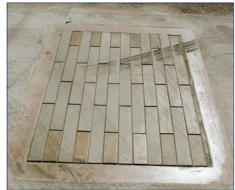
Skid marks on top of pavers show evidence of deliberate attempts to disturb installation. The mortar-set Narrow Modular Pavers held fast and were not dislodged by vehicular traffic.
